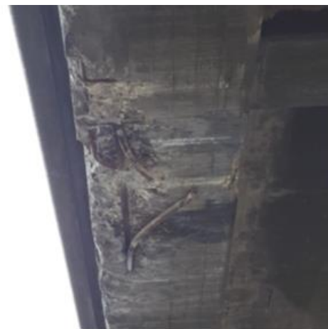
Figure 13. Photograph of the edge beam damage
