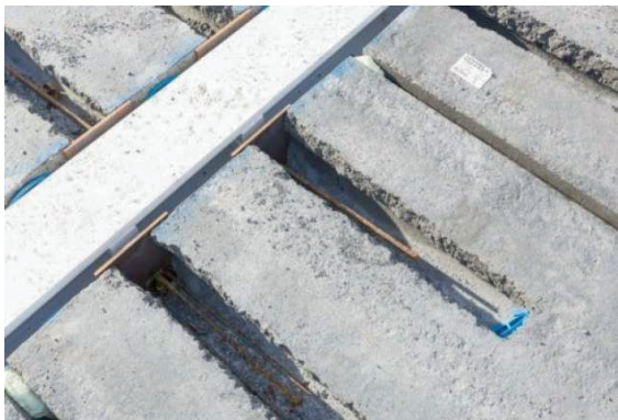
Figure 2.5 | A wet (grouted) 'demountable' connection between a hollow core slab and an integrated steel beam in the temporary Amsterdam court house (Cepezed Projects).
