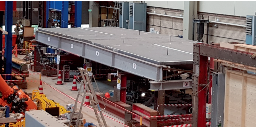
(e) Final assembly. The rods extending from the top surfaces of the floor elements were used for hoisting.
