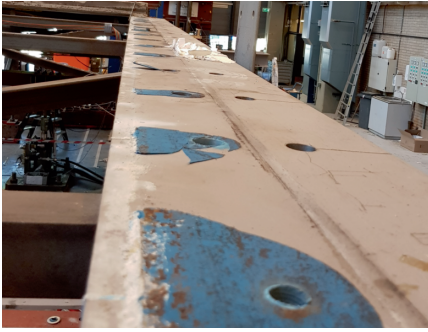
(a) Removal of the floor elements revealed substantial epoxy resin leakage at the steel-concrete interface.
