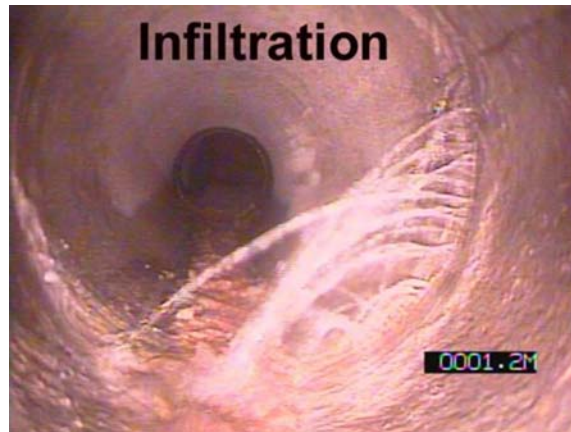
Figure 3.47 Clear example of infiltration of groundwater into a sewer pipe. Source: Deltares.
